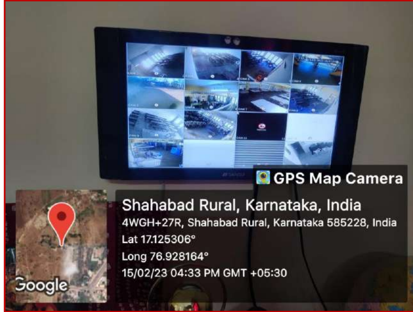
CCTV Camera Surveillance
